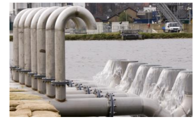
...maintaining a safe and reliable water supply
