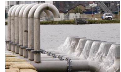
...maintaining a safe and reliable water supply
