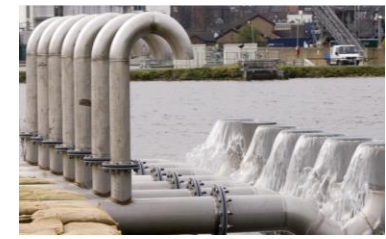
...maintaining a safe and reliable water supply
