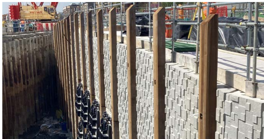
Costain VINCI Construction Grands Projets and Bachy Soletanche JV Thames Tideway East project. The NbS design on the river wall provides a shelving pattern that will allow moisture to be retained, increasing the habitat available for target species within the tidal River Thames.
