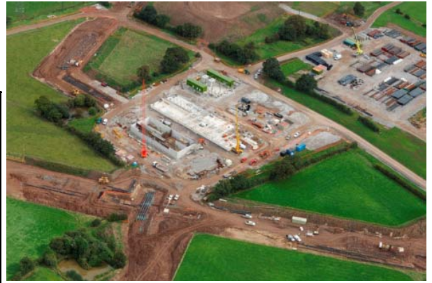
The GDF Gas Storage project at Stublach, currently in construction. View of the Solution Mining Compound
