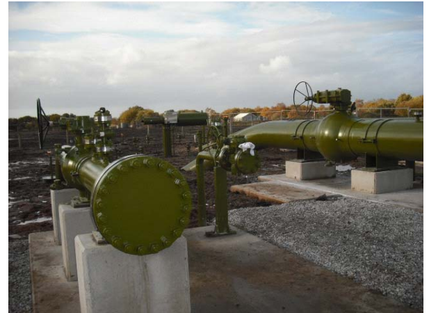
The E.ON Gas Storage project at Holford. Gas pipelines complete and Gas Plant in detailed design.
