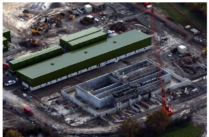
View of the Pumping House with the degassing tanks in the foreground under construction at Stublach Brine and Water Facility
