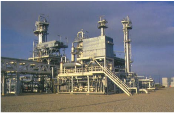
Figure 2. Teesside Gas Processing Plant Train 1 DRIZO Unit.
