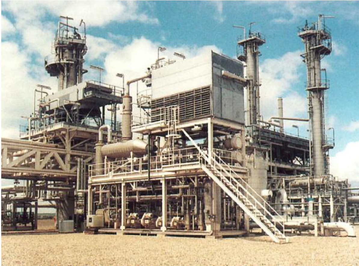
Figure 2 - DRIZO® TEG Regeneration Module at px Teesside Gas Processing Plant
